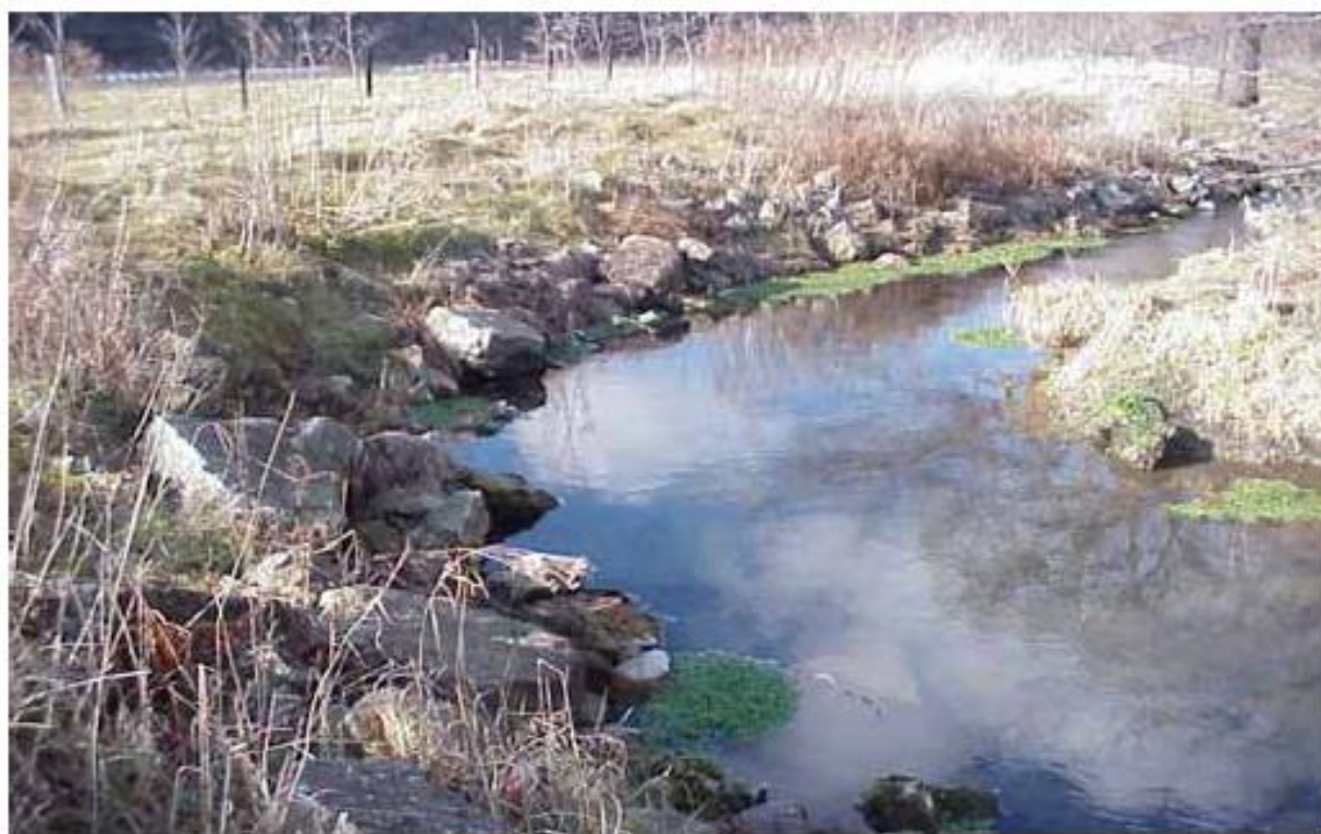
Figure 20. Riprap along the bend of a stream with vegetation between the rocks
