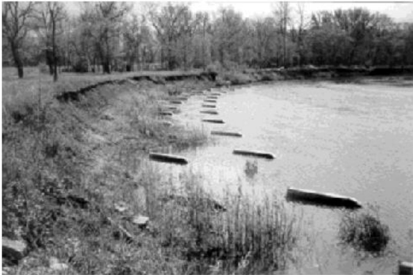
Figure 26. Replacement of sediment on bank from Vanes
