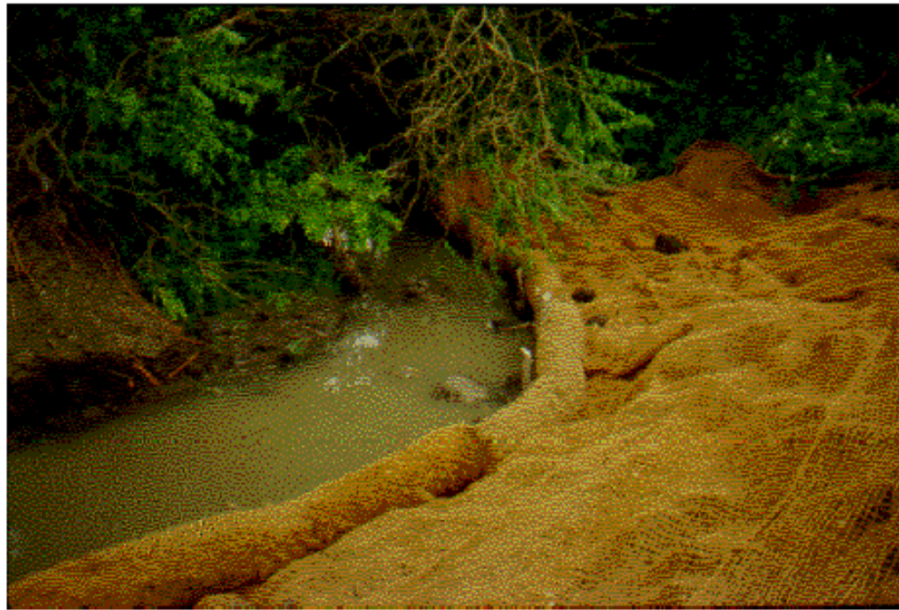
Figure 15. Coconut roll staked to bank with coconut fiber fabric across slope to protect exposed soil
